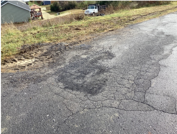
2004 asphalt pavement pot hole formation
